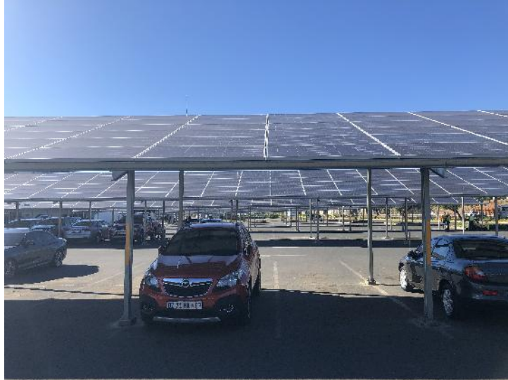
Figure 5: Photo of parking bays covered with solar PV generation in Johannesburg, South Africa
