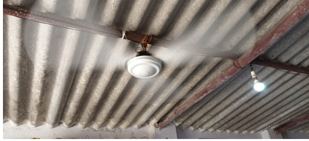
Figure 10: A BLDC fan in action
